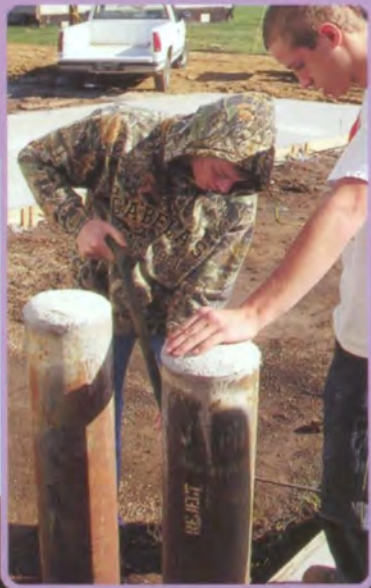
Ethan Larson and Chris Smith get ready to pour concrete for a driveway at the new community building in Highland. Both Ag Mechanics classes helped out by doing everything from laying bricks to putting up drywall.
