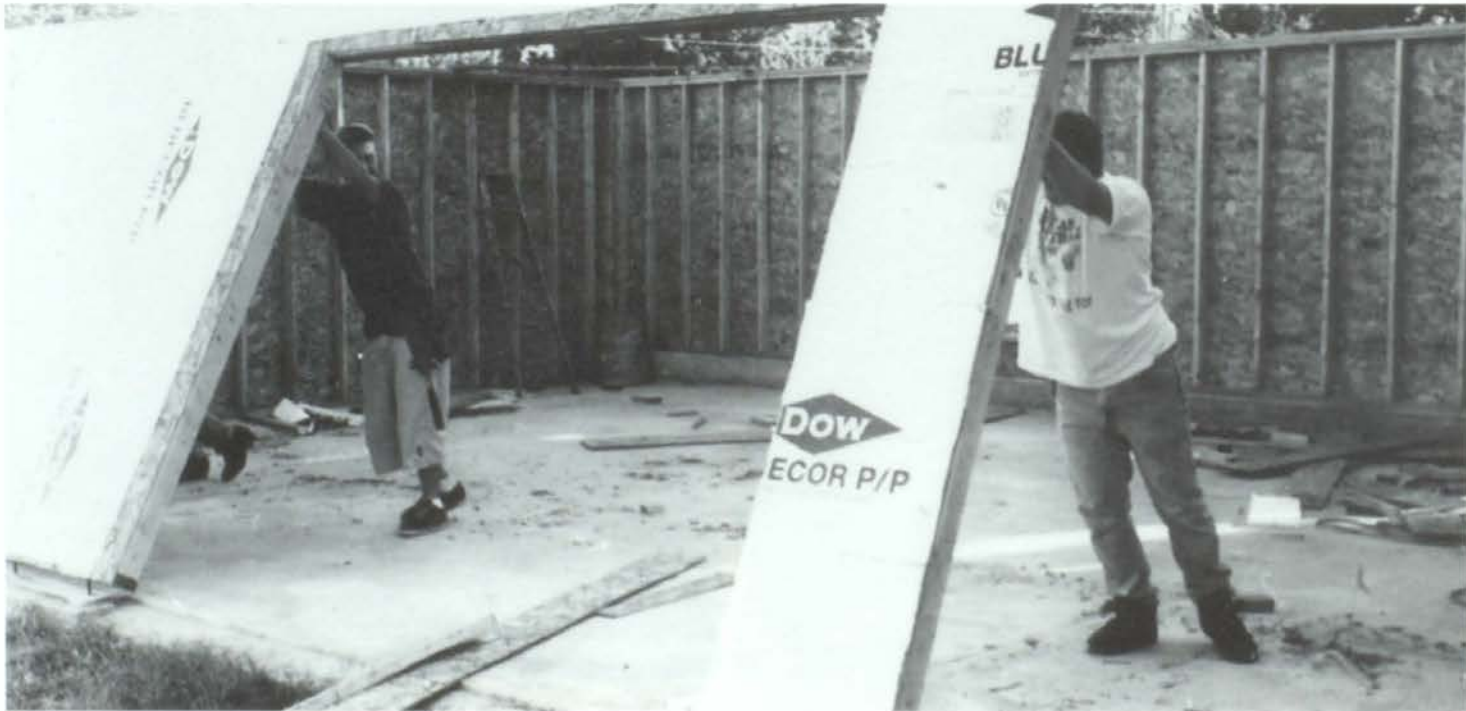
Tim Uplinger and Matt McKittrick erect the west wall of the Building Trades' garage. Matt and Tim both worked on the garage during their Building Trades and advanced industrial arts classes. Photo by Jamie Christenson.
