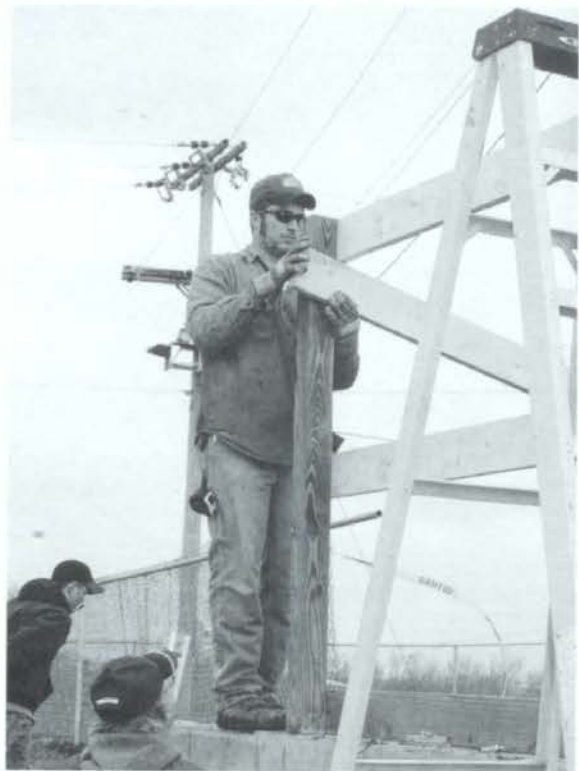
Above: Wade Sutton lines up support beams on the new addition to the bus barn while Mr. Velharticky supervises. Photo by Casey Beemer
